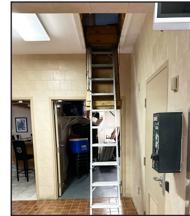
Central storage space for gear and equipment is accessible through residential-style attic access ladder in kitchen.
